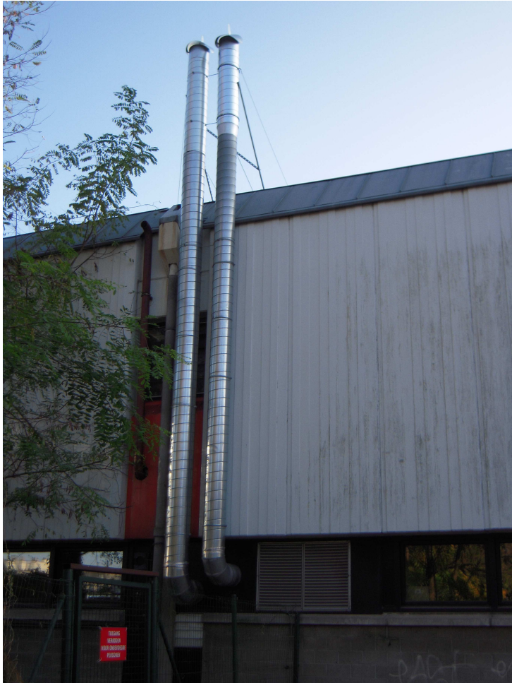
Figure 3.37: The ventilation and exhaust gas stack were heightened to prevent EGR.
